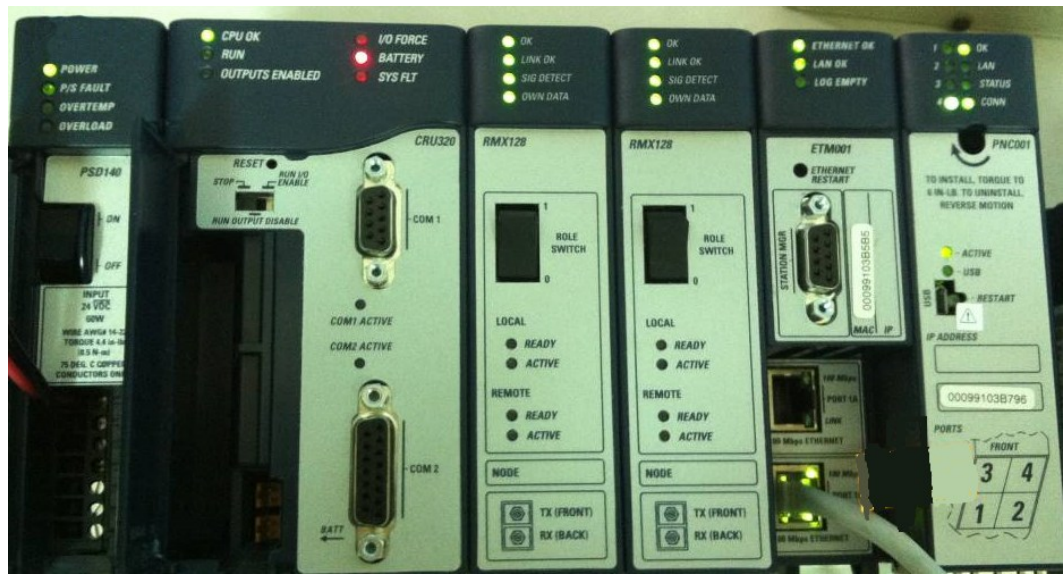
Figure 10: Current Rack Configuration
