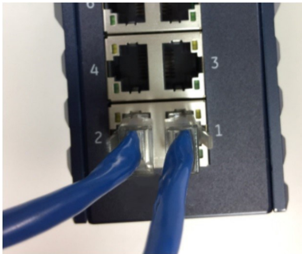
Figure 11: Ports 1 & 2 Copper Connections
