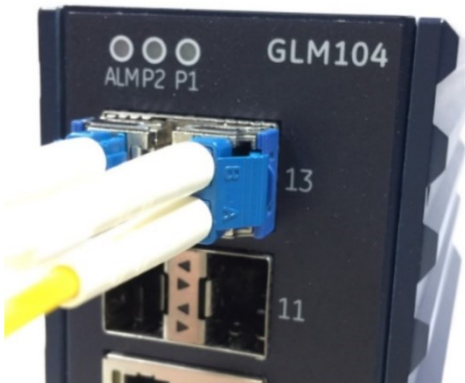
Figure 15: Attach Fiber-Optic Cables to Installed SFP Socket
